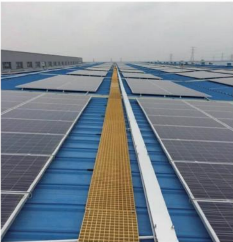
FRP Rooftop Walkway
